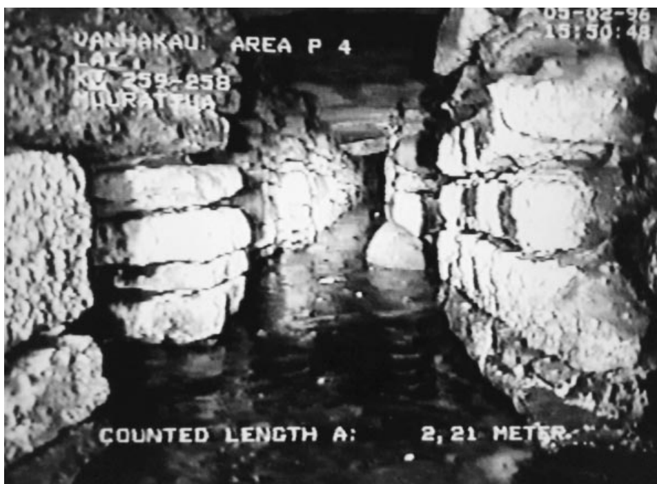
Integrating old and new sustainable technology. The sewers built in the 18th century in the Old Town of Tallinn are still actively used. These sewers are now renovated with the help of videos taken by a robot camera operated with a remote control system. Photo: Tallinn Water Ltd/Instituform Finland Ltd.
